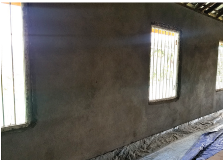
Completed portion of wall plaster in Alison House second floor. Window reveals to be done.
