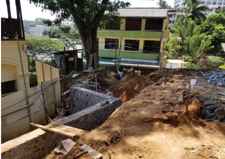
Rubble Retaining wall RW6 on Gaster end .of Commerce Block. Plinth beam to cast on top of the wall
