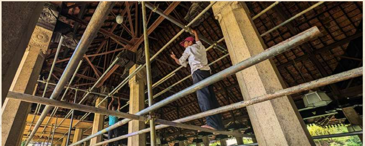
Image above: Restoration work in progress - of the pekada on pillars at the right-side nave of the Chapel
